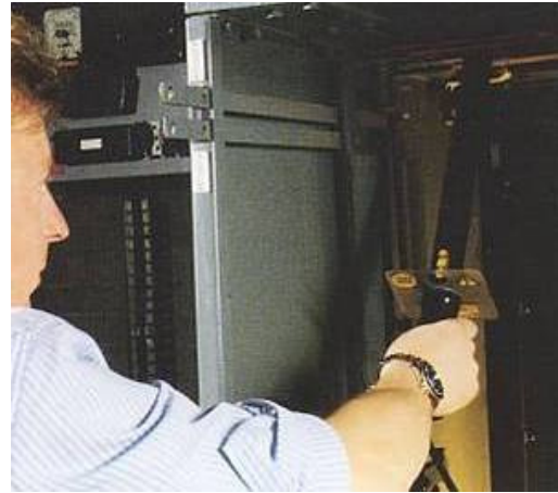
HVI - Switchgear Testing
